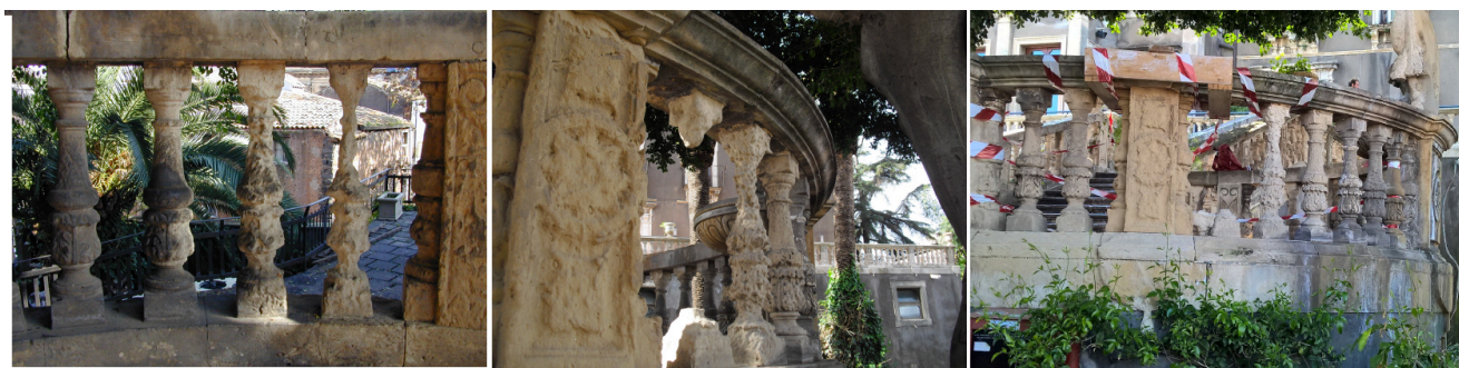
Fig.16: Three stages of decay: on the left photo of 2001; in the centre, the baluster without spindle (February 2015) and on the right, collapse of the capital and of the handrail overlying (May 2015)
