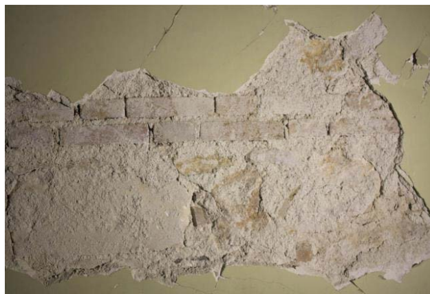
Fig. 3: The muratura listata visible thanks to the detachment of the plaster
