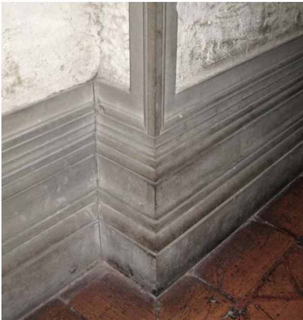
Fig. 2: Lower part of the pedestal profile in the Ricetto of the Biblioteca Laurenziana
