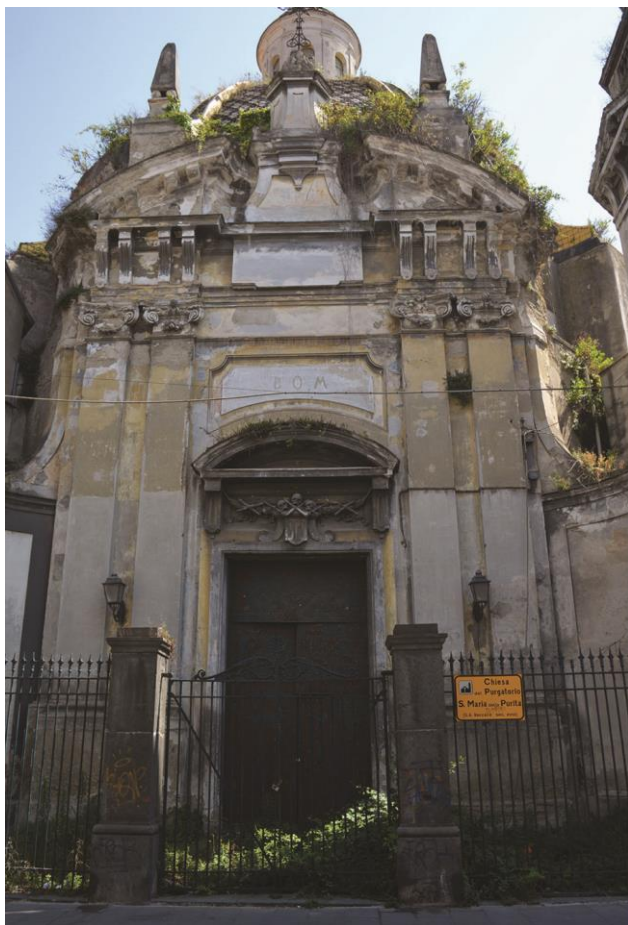
Fig. 1: Degrade conditions of the façade of the church of Santa Maria della Purità. Photography by Mario Ronca.
