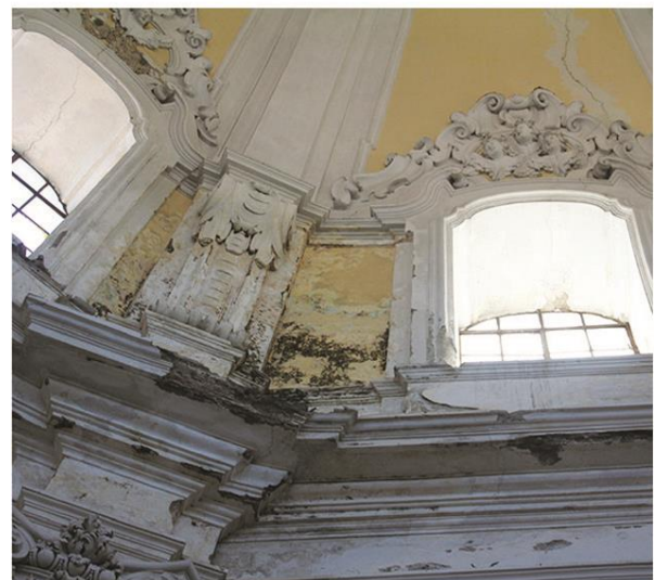
Fig. 2: Degrade conditions of the extrados and intrados of the dome. Photography by Mario Ronca.
