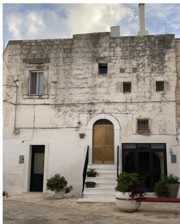
Fig. 3: Example of the state of decay of an external wall of a building, featured by crusts, dampness, and degradation of tuff blocks along the exposed surfaces
