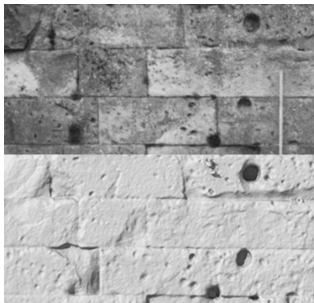
Fig. 4: Comparison between the state of preservation in the 20s (photo on the top, year 1925) and the actual 3D surface (3D model on the bottom, February 2024) of the city wall; detail detecting the differences on the left tufa ashlar, nowadays partially missing probably due to the impacts visible in the photo that contributed to deteriorate the stone. Credits: Top, as Fig. 3; Bottom, model by S. Bertacchi.
