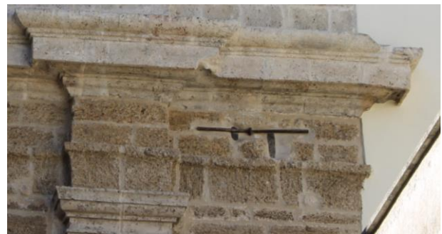
Fig. 36: Detail of key head of the chain after completion of the works
