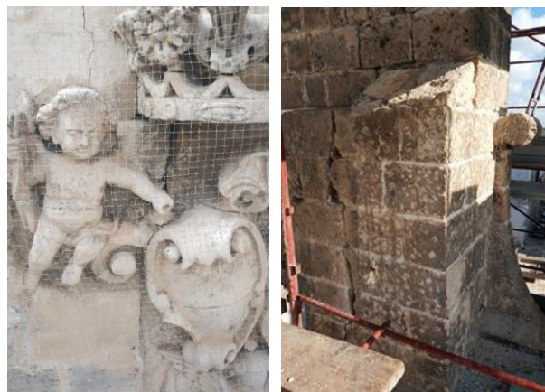
Fig. 27a-b: Cracking on east and ovest elevation
