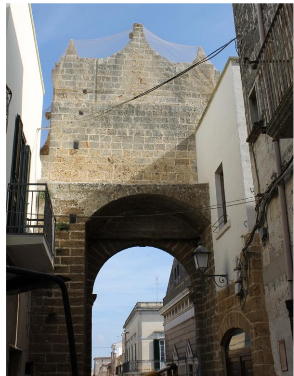
Fig. 21: Ovest elevation, towards Via Martiri della Libertà, state of the site before the intervention
